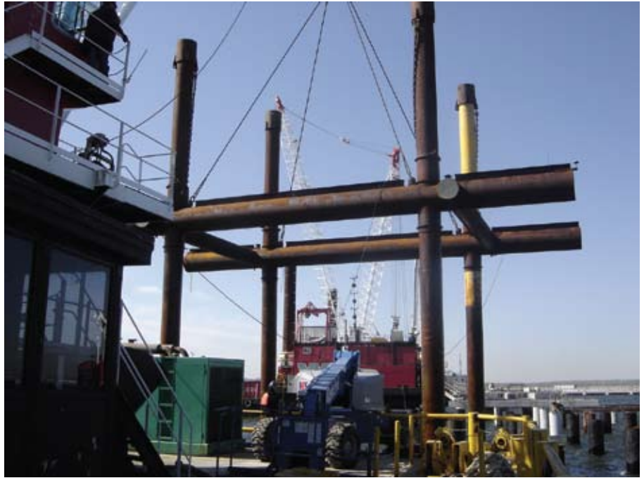
The Weeks #532 Derrick lifts the 70-ton pile driving template platform base complete with temporary support piles.
