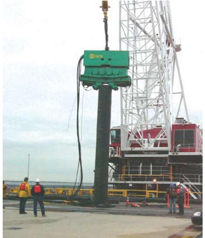
Trestle 3A test pile program: The Weeks #532 Derrick drives a 42" dia. x 3/4" w.t. open-end pipe pile through a cutout in the old Trestle 3 concrete deck, with an ICE 125 vibratory hammer.
