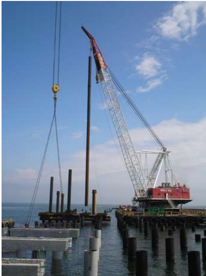
(Right) Weeks #532 Derrick sets 175ft long 42" dia x 3/4" w.t. pipe pile in template platform frame (Left) Weeks #720 jackup barge sets a 30-ton precast pile cap on jacketed piles.
