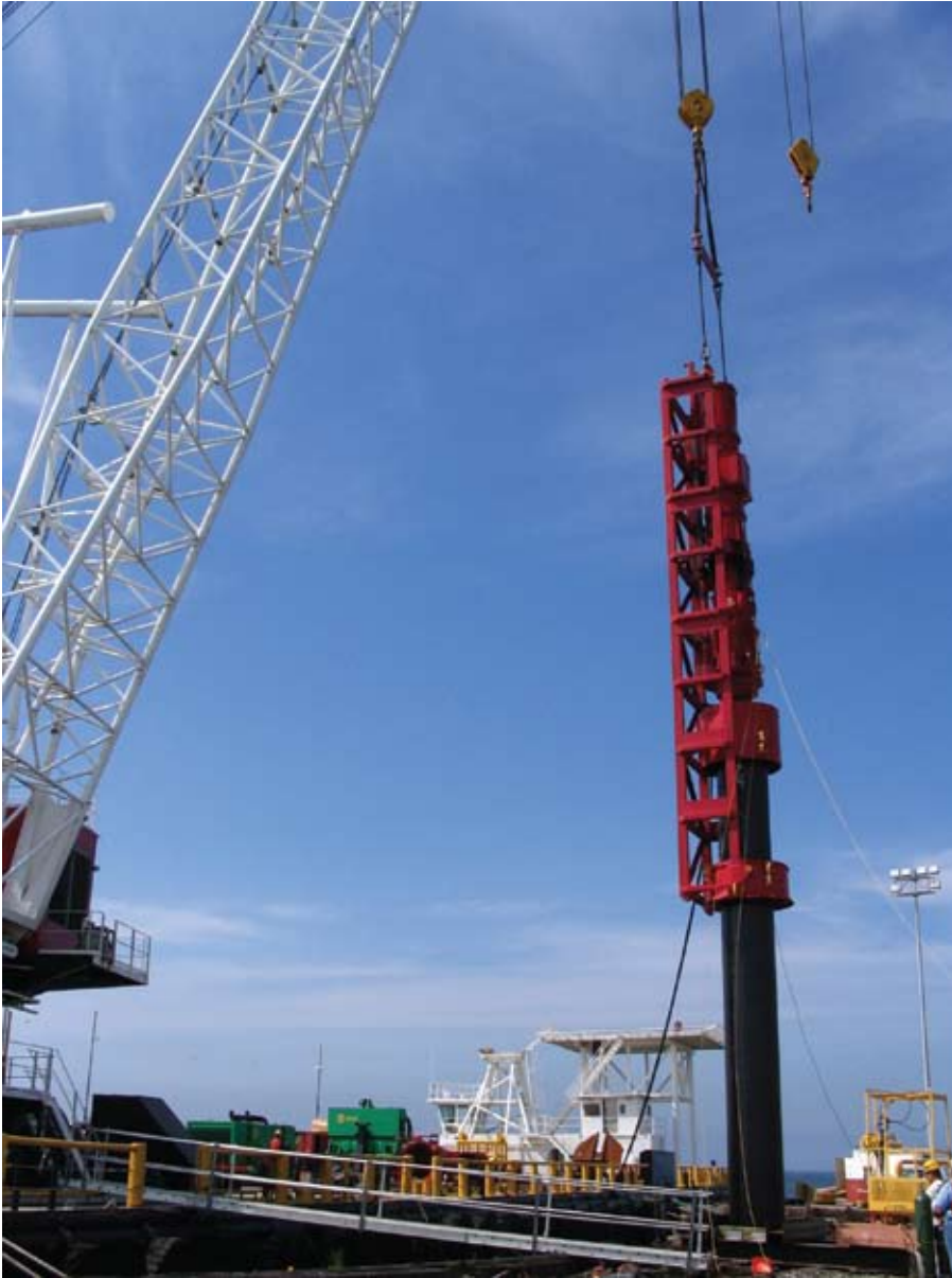
The Weeks #532 Derrick drives 42" x 3/4" w.t x 158-foot test pile "K25" with the Pileco D-125 diesel impact hammer.
