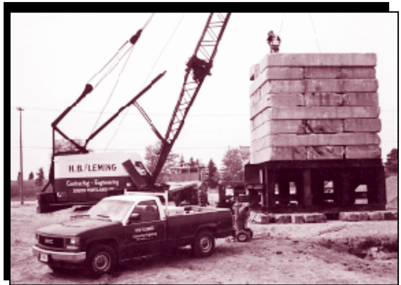
An LS-109 crawler crane finishing the erection of the concrete blocks for a static load test of a 100-ton HP 12 x 53 steel pile.
