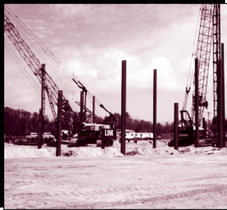
LS-118 and LS109 crawler cranes driving HP 12 x 53 piles for a Home Depot in Portland, Maine. The pile hammer is an ICE 42S diesel.
