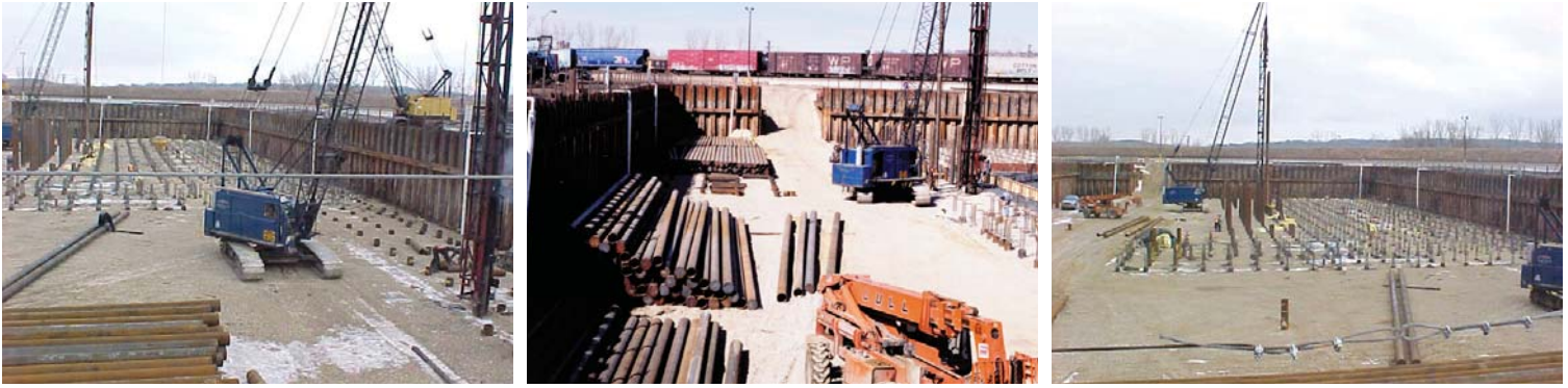
Pile were delivered from the mill by rail in lengths that had been determined by the pre-production pile-testing program.
