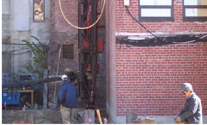
The project involved driving piles in an historic area where building owners can be “sensitive” to vibrations.
