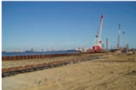
The HZ and AZ combi-wall completed with anchor wall and tie-rods installed.
