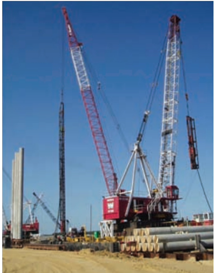
Four 36" diameter cylinder piles wait to be driven by a Raymond 40X hammer hoisted by the Weeks 541 crane barge.
