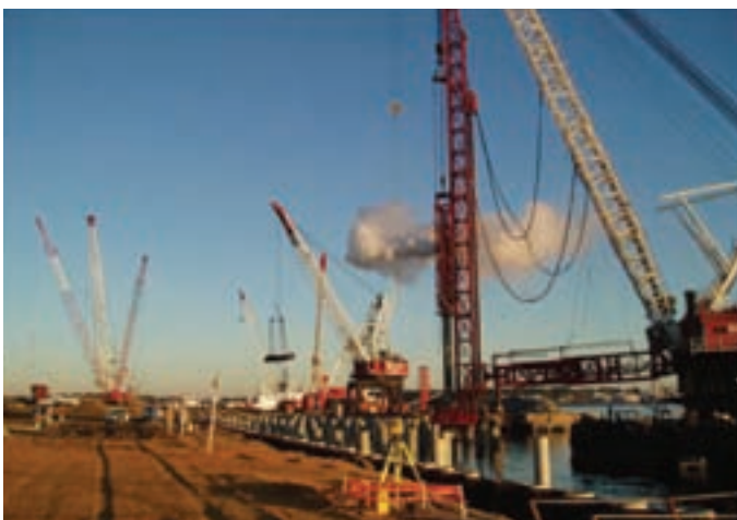
The Weeks 526 and Raymond 60X steam hammer completes the driving of a 36" diameter concrete cylinder pile.
