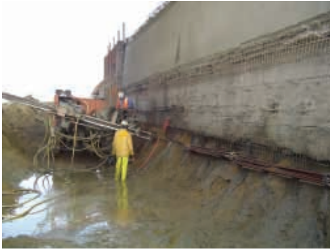
Soil nail system used to create a surface that resembles rock. The company pounds soil nails into a rock surface and adds mesh and spray grout to create a concrete wall that has a natural rock look.
