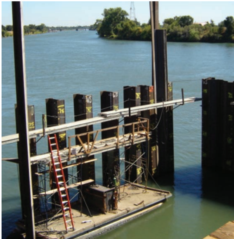
Figure 3: King piles were placed precisely to accommodate the hot-rolled steel sheet piling
