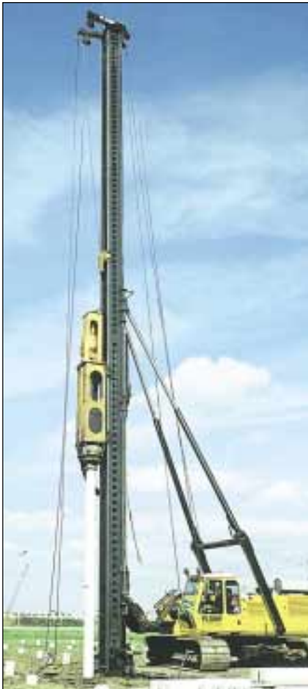
PVE Model 5021-S driving 12" pre-stressed concrete piles with a Pilemer Model DKH-5L Hyd Impact Hammer rated at 43,398 ft./lbs.
