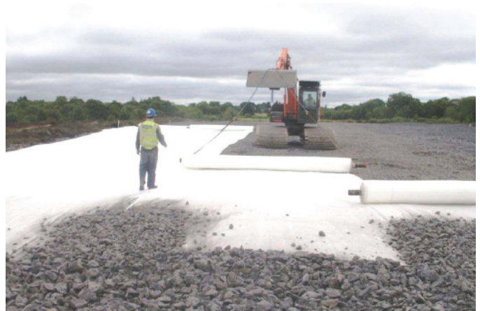
The weight of these machines and the uneven surface of the temporary platform caused a significant amount of vibration across the site.
