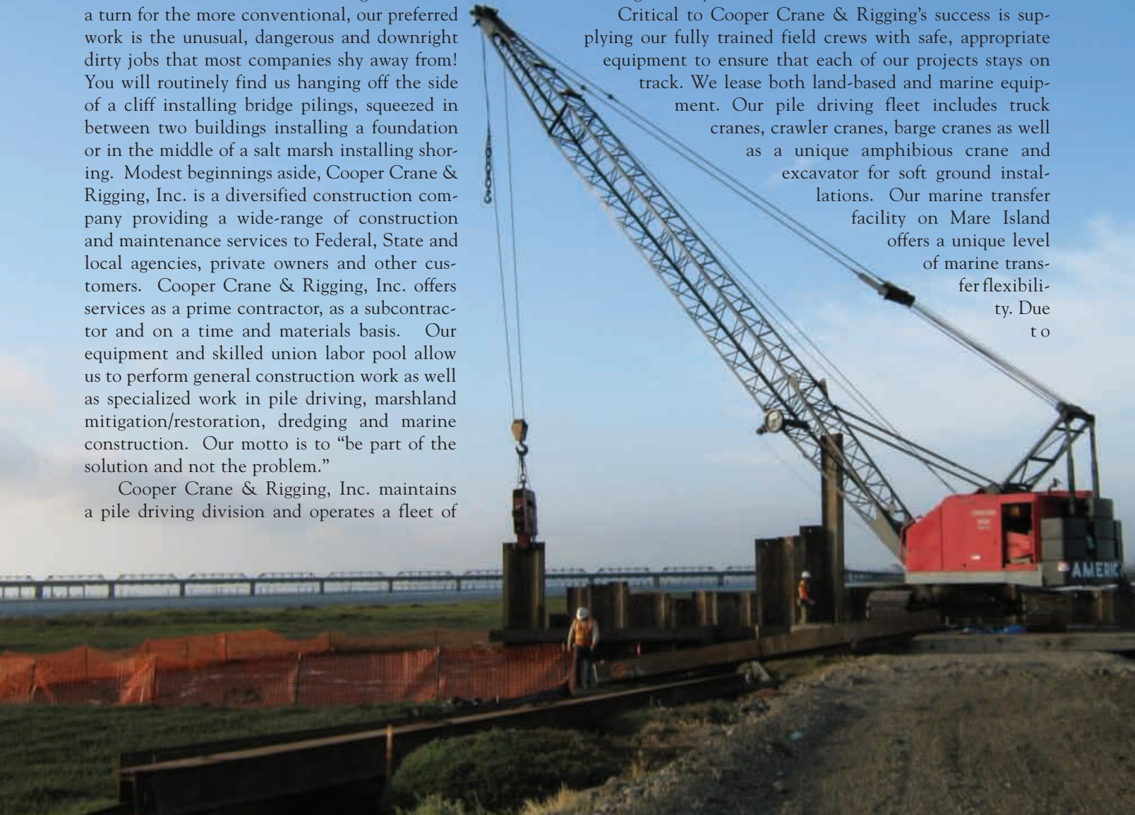
Installation of a cofferdam at Don Edwards San Francisco Bay National Refuge, Pond SF2, CA.
