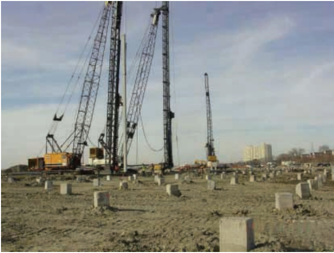
This 25 acre site is situated on the Elizabeth River and mainly produces square piles and double tees.
