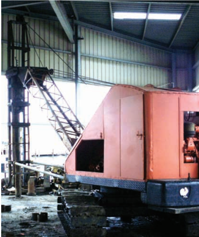
There was very little room for error and great precaution had to be taken not to damage the existing buildings.
