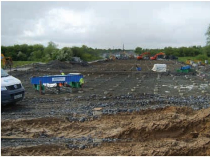
One of the main obstacles was the volume of site traffic passing in heavy earthmoving vehicles.
