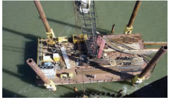
Figure 6. Jack-up Barge at Morris Island Lighthouse (taken from on top of lighthouse).
