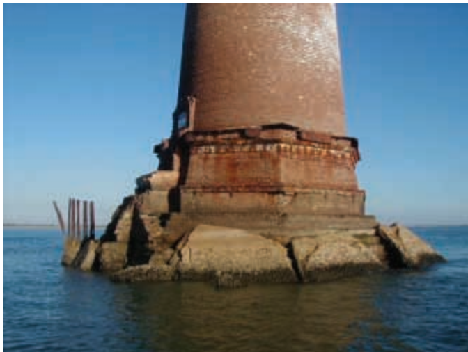
Figure 13. 1939 wall cap remnants
