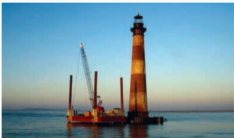
The Pile Driving Contractors Association 2009 Project of the Year - Greater than $2 Million.
