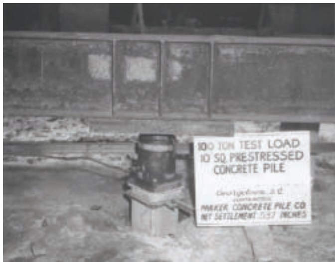
1963 - Georgetown, SC 100-ton static test load on 10-inch prestressed pile. Helped legitimize prestressed with regional design professionals.
