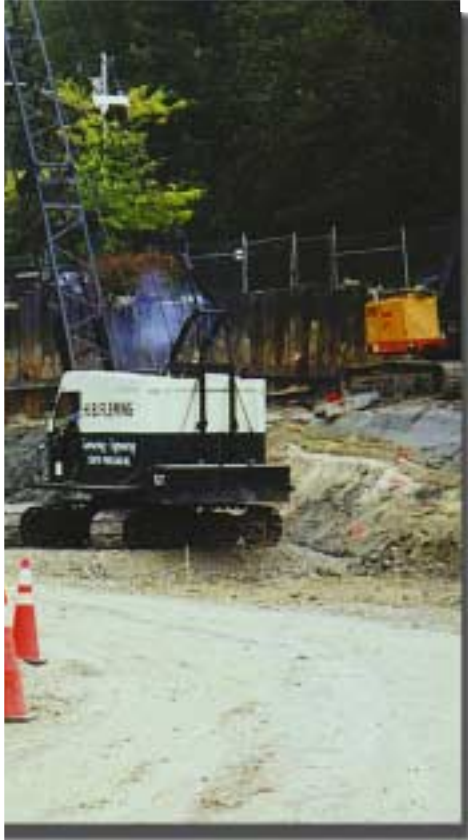
H.B. Fleming installs #8 sheet pile with Helical Anchor tiebacks for the Maine Medical Center in Portland, Maine.
