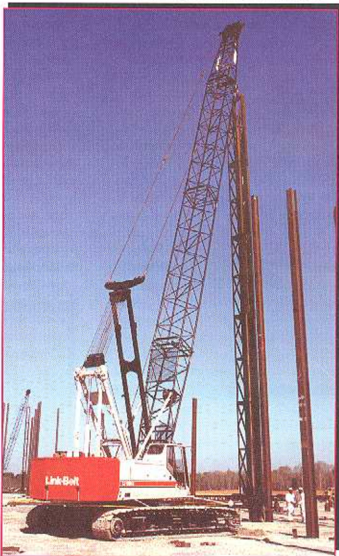
A Link-Belt LS-138 H II at work at the Honda Manufacturing Plant in Lincoln, Ala.
