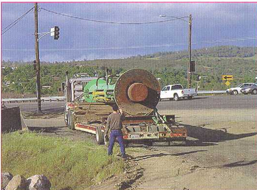
The LMC 50 hydraulic impact hammer, designed and built by Lucas Marine, is delivered to the Putah Creek job site.
