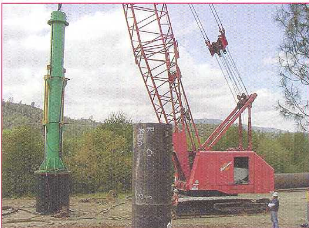
Lucas Marine's LMC 50 hydraulic impact hammer driving a 60-inch pile for the Putah Creek bridge.
