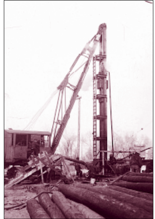
A Northwest Crane drives timber piles in Eastern Colorado for Lawrence Construction in 1935.
