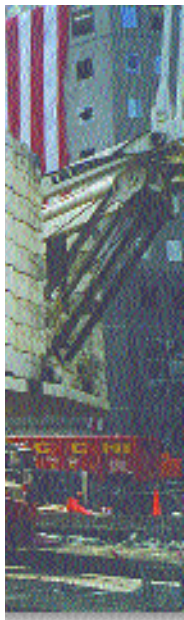
A 700-ton Leibherr operates from West Street. Thirty-eight truckloads delivered the crane to the site.
