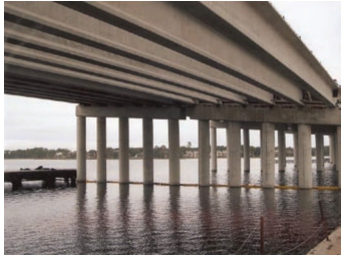
54" concrete cylinder pile in place with the concrete cap and prestress beams set.
