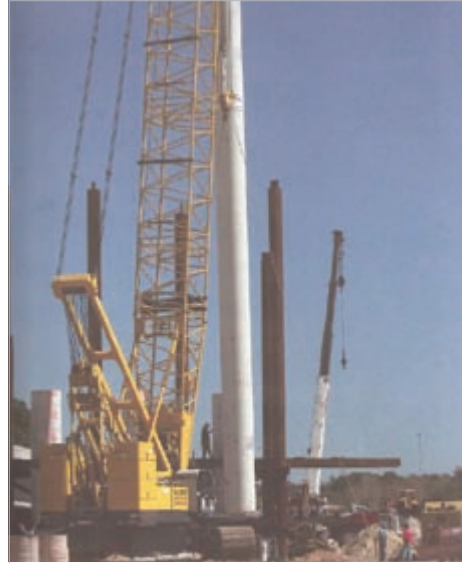
54" concrete cylinder pile in place with the concrete cap and prestress beams set.
