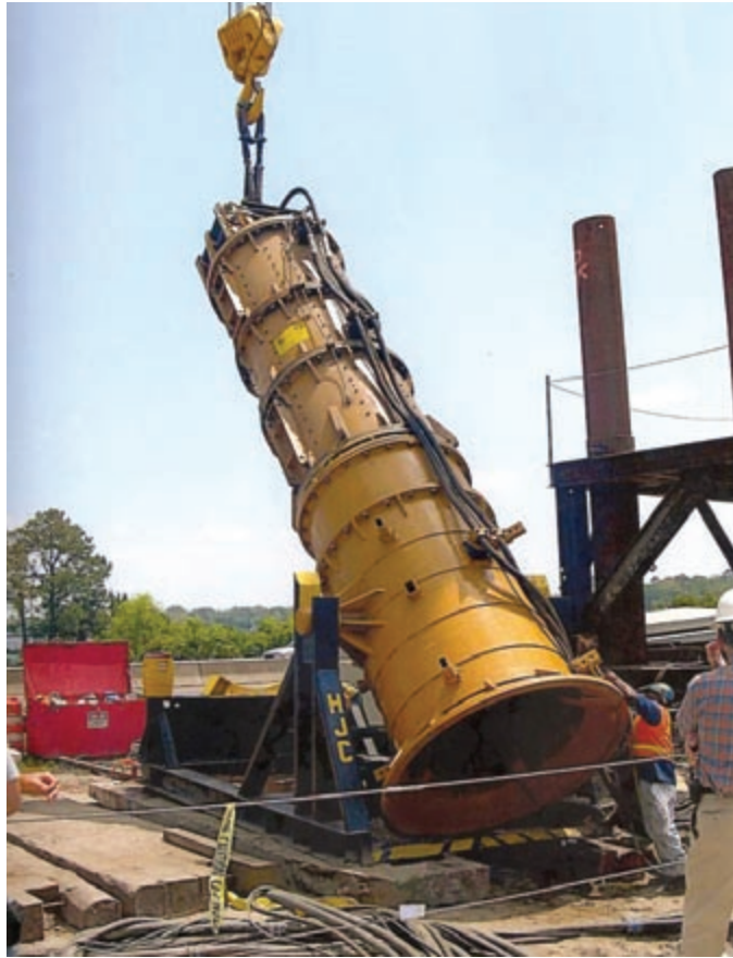
LEFT: APE 400 Hydraulic Impact Hammer being lifted from the rack to drive 54" pile.
