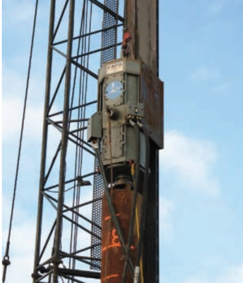
The 140 kW (200Hp) Resonant Driver mounted on a 600 mm diameter pipe pile
