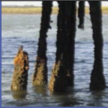
Wood Pilings Rot.
