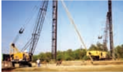
Timber composite piles being driven for Wal-Mart Super Store in Harvey, La.
