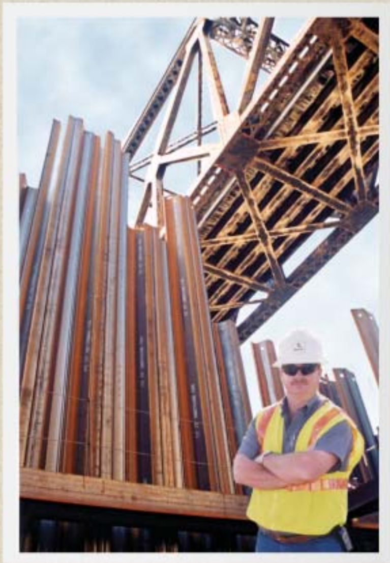
Dallas DART Pilot Project by Austin Bridge & Road Over the Trinity River
