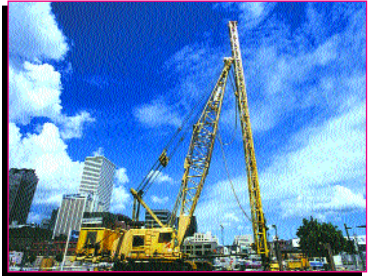
A Boh Bros. Construction crew at work at the Energy Center parking facility in New Orleans.
