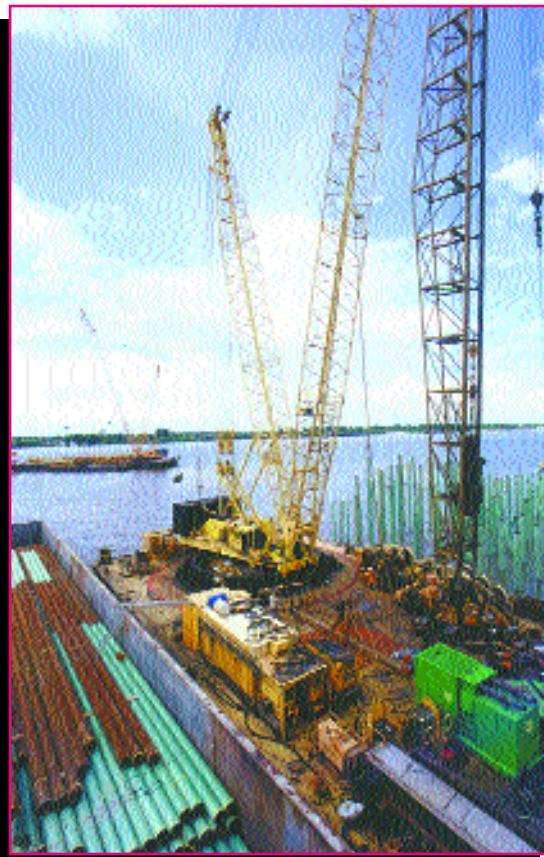
Boh Bros. has done work at the Napoleon Ave. wharf at the port of New Orleans.
