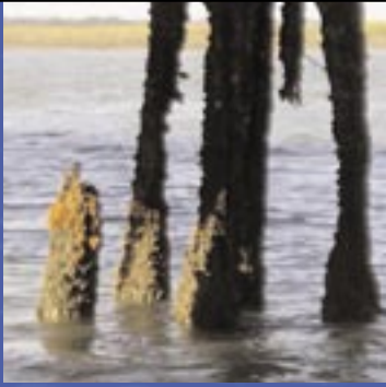
Wood Pilings Rot.
