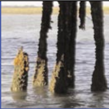
Wood Pilings Rot.
