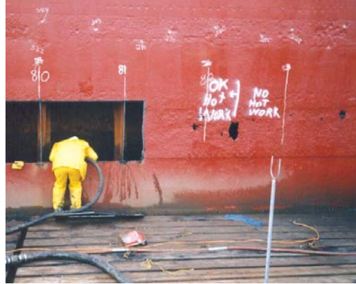
The hull of the 62-year old battleship had corroded extensively from resting at the bottom of the Mobile Bay for nearly four decades.
