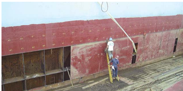
D.R. Jordan, president of Jordan Pile Driving, Inc., says steel sheet piling was used as shoring to allow excavation alongside the ship’s hull to expose deteriorated steel that was then removed and replaced.
