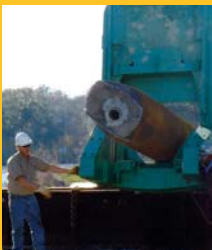
OFFSHORE RESULTS Demolition of offshore oil platform & underwater pipeline with concrete jacket
