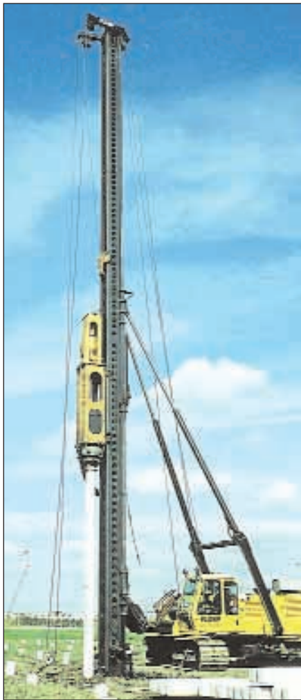
PVE Model 5021-S driving 12" pre-stressed concrete piles with a Pilemer Model DKH-5L Hyd Impact Hammer rated at 43,398 ft./lbs.
