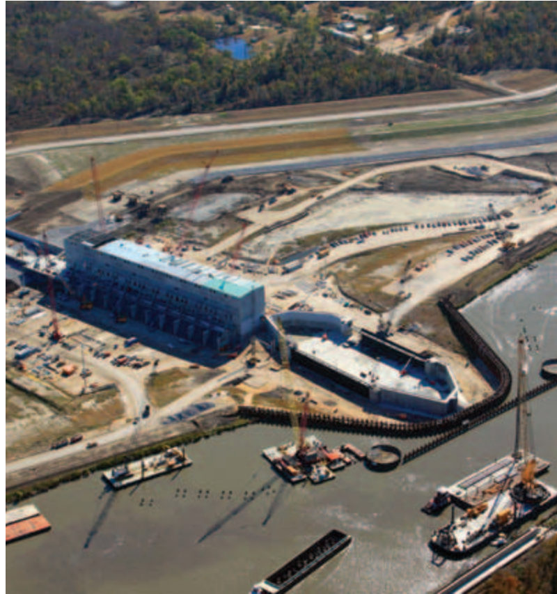
Fugro provided inspection, load testing, and NDT Services for the New GIWW Closure Project.
