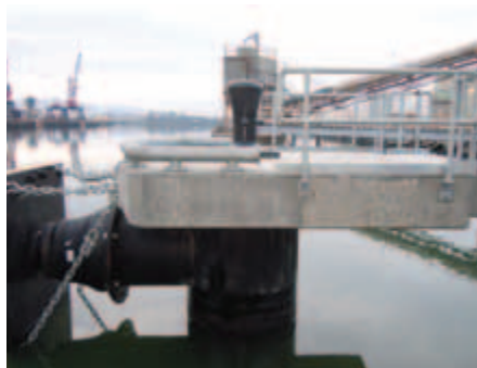
A close-up version showing the placing/guiding of the monopile into the template.
