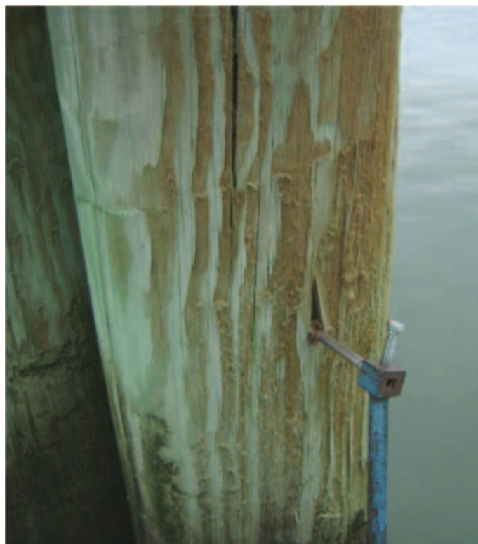
Figure 1 (Left): Pilings in Charleston, SC, damaged by salt exposure. This piling was located in a marina and subjected to frequent wetting and sea-spray.
