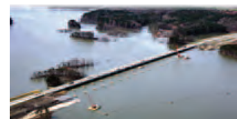
On the Cover: Aerial East Bound and Existing Pier Caps for the 1-80 Widening over the Meander Reservoir by The Great Lakes Construction Co. (submitted by Jeremy Levenson and Randy Radel, GLC)
