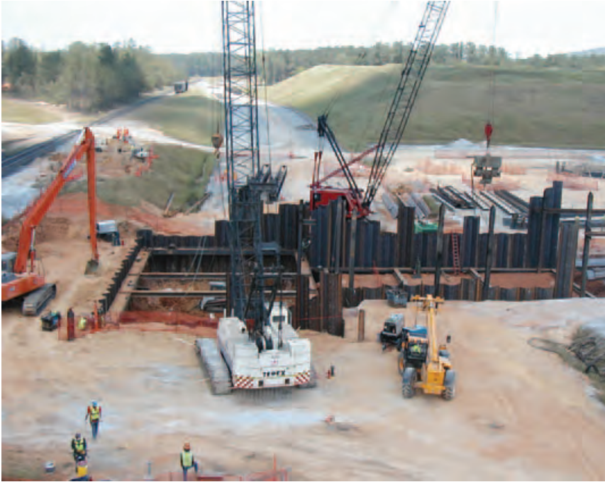
Sheet piles and interior bracing for rail unloading (left) and conveyor tunnel (right).
