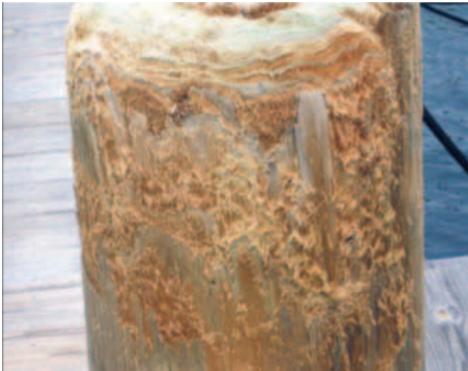
Figure 2. Salt killed piers, pilings, seawalls, and other marine structures are common.
