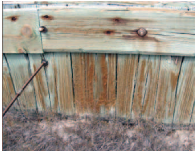
Figure 3. Salt kill occurs as intertidal salt from the water is deposited on the wood structures or wicks upward in the wood.
