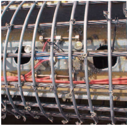
Vibrating wire strain gages (weldable mounts on an steel stinger and an embedment mount tied to a prestressing strand) installed in a PSC pile prior to concrete placement.
