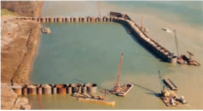
This cofferdam is part of the Omsted Lock and Dam project. While replacing locks and dams on the Ohio River, the team drove and installed more than 21,000 tons of sheetpile.
