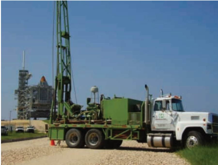
Installation of test piles, NASA Lightning Protection System at Launch Pad 39B
