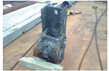
Figure 7. 10-inch Pipe Horizontal Brace
