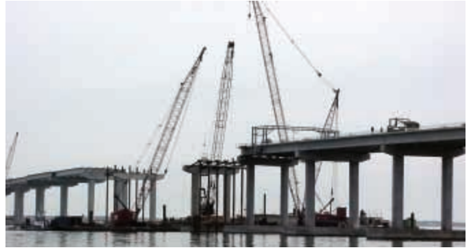
Balfour Beatty Infrastructure, Inc. workers drove 2,400 number 762-millimeter square piles weighing up to 60 and 70 tons each as part of the Virginia Dare Memorial Bridge project over Croatan Sound in Manteo, North Carolina. Shown here is a completed high-rise section in the bridge center, supported by up to 60 piles in each bridge footing.
