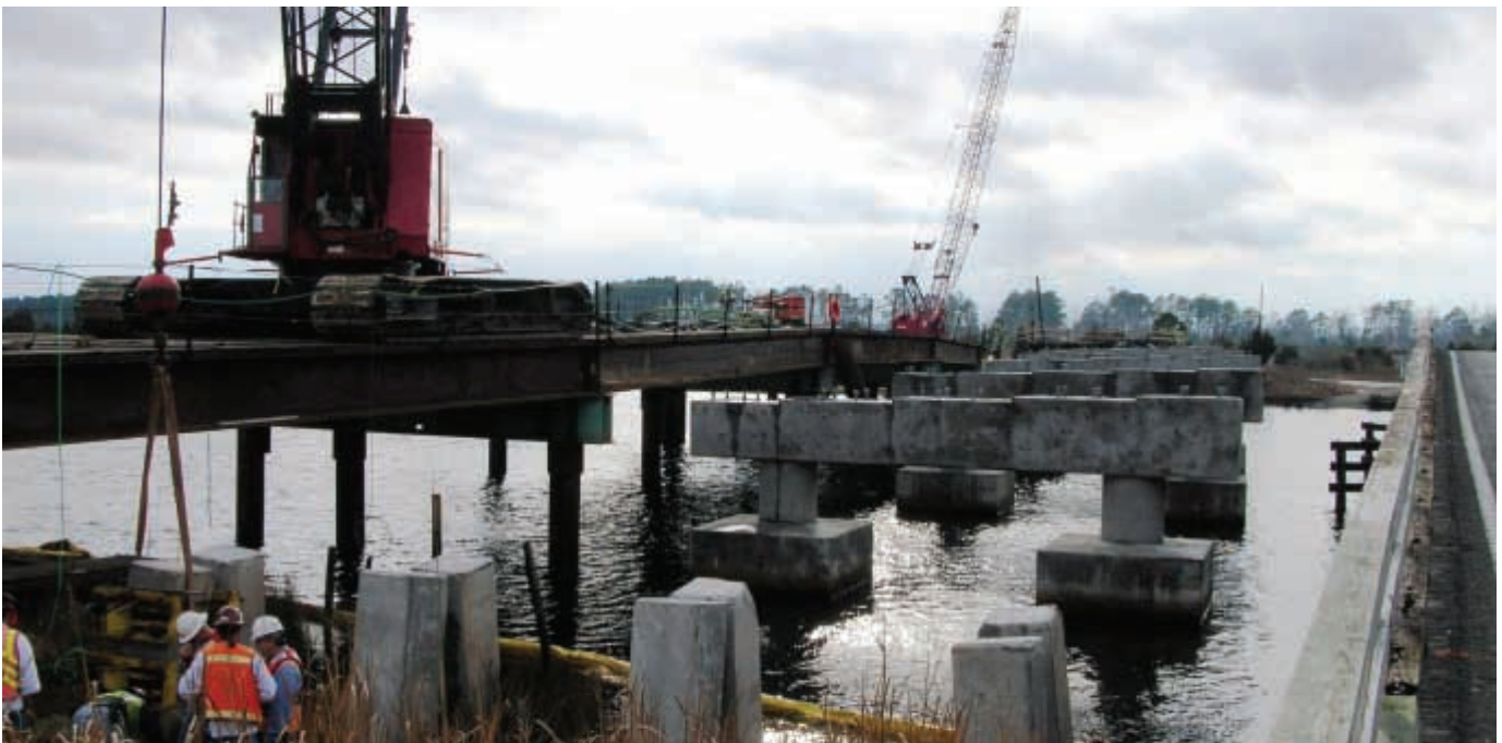
The White Oak River Bridge called for steel pipe pile, concrete pile with steel pile stingers in a highly sensitive wetlands area near Stella, North Carolina. Pictured here are low-water footings supported by 24-inch OD metalized pipe pile.
