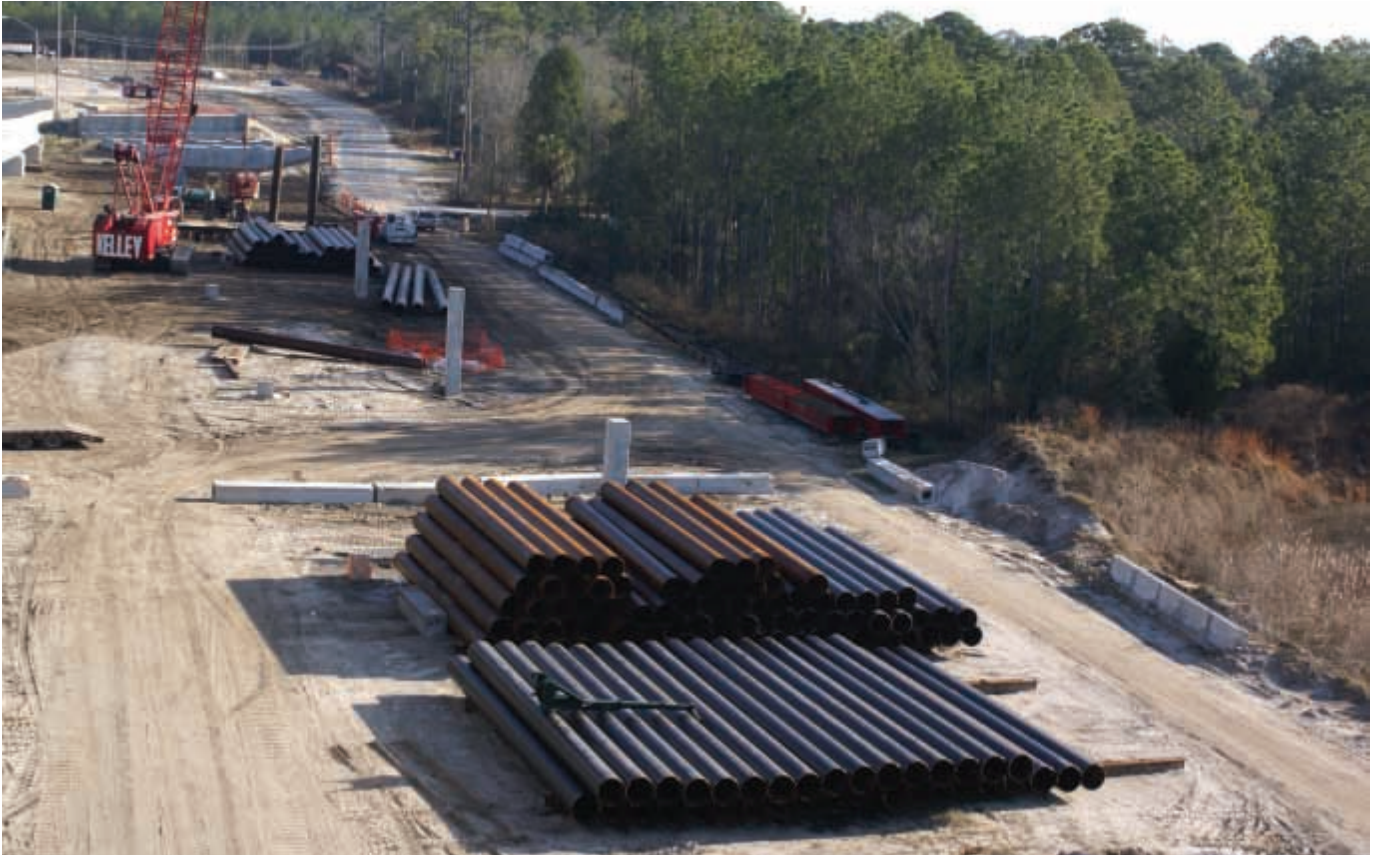
Over 40,000' of 30" diameter heavy wall pipe replaced failing concrete piles during construction of the Bay Bridge near Panama City, Florida.
