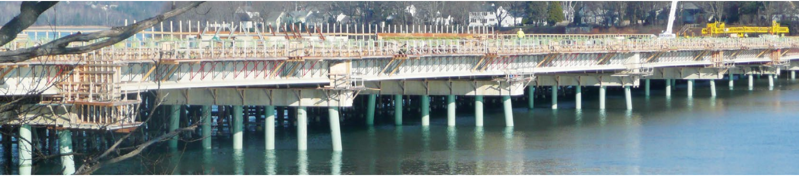
Martin's Point Bridge nearing completion. A few of the 10 piers are shown.
