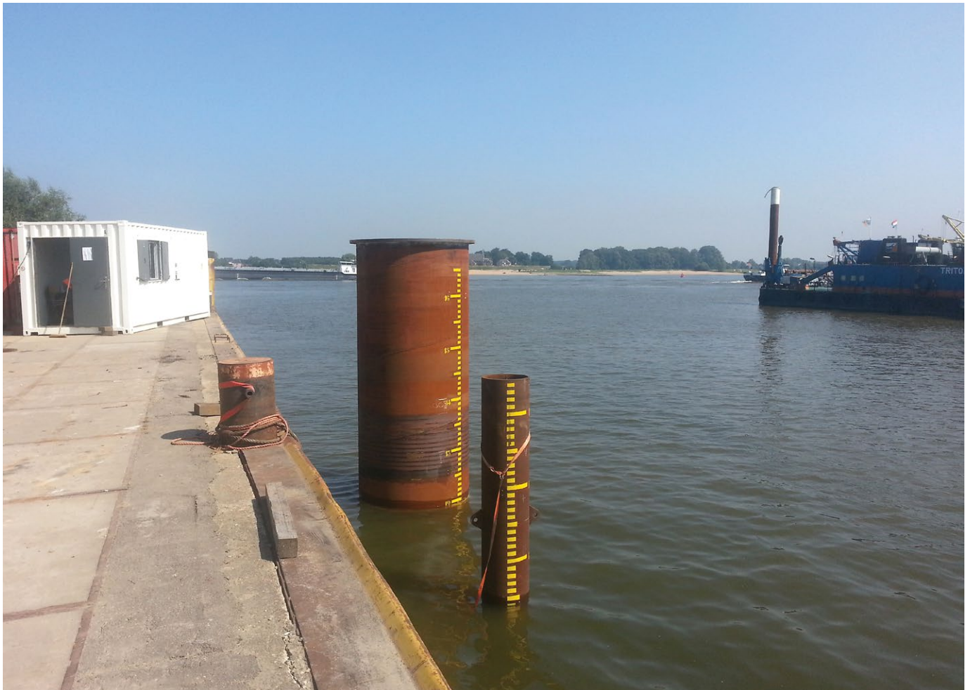
The result of near-shore tests in August 2013; two piles (one 2.2 metres and one 0.7 metres in diameter) driven using BLUE Piling Technology
