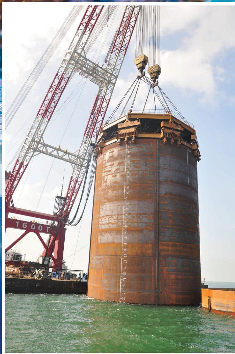
RSC Bio Solutions' products were used during the construction of the Zhuhai-Macau Bridge in China by APE
