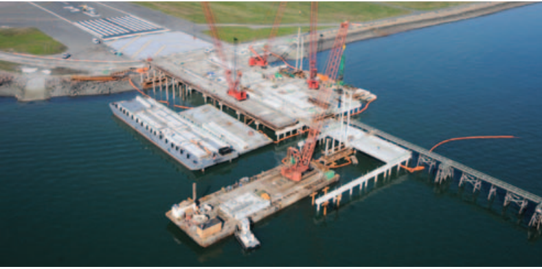
September 2011: Aerial view of two Manitowoc 999's driving 18 square piles on the three line, one Manitowoc 2250 driving piles on the water, and the fourth Manitowoc 999 unloading barges.
