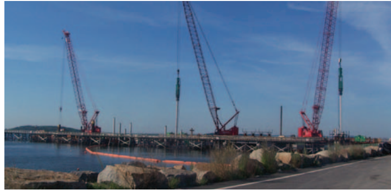
All cranes and barges have to be moved off or away from the deck nightly.
