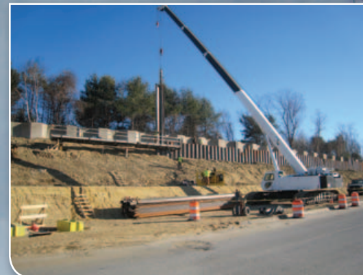
Working on the permanent retaining wall for the Massachusetts Department of Transportation in Newburyport, Mass. was a $1.5 million project for Sea & Shore Contracting
