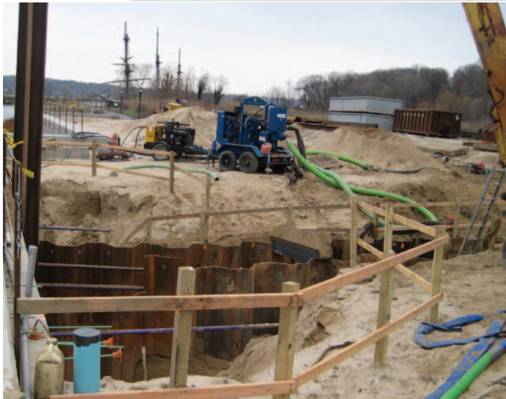
Above: Steel sheet piling (40 feet long) was necessary to support the excavation for a storm drain pipe that passed through the new bulkhead at 10 feet below Mean Low Water (MLW). A SSP cofferdam (not visible in photo) was employed on the outside of the new bulkhead to control the seawater.
