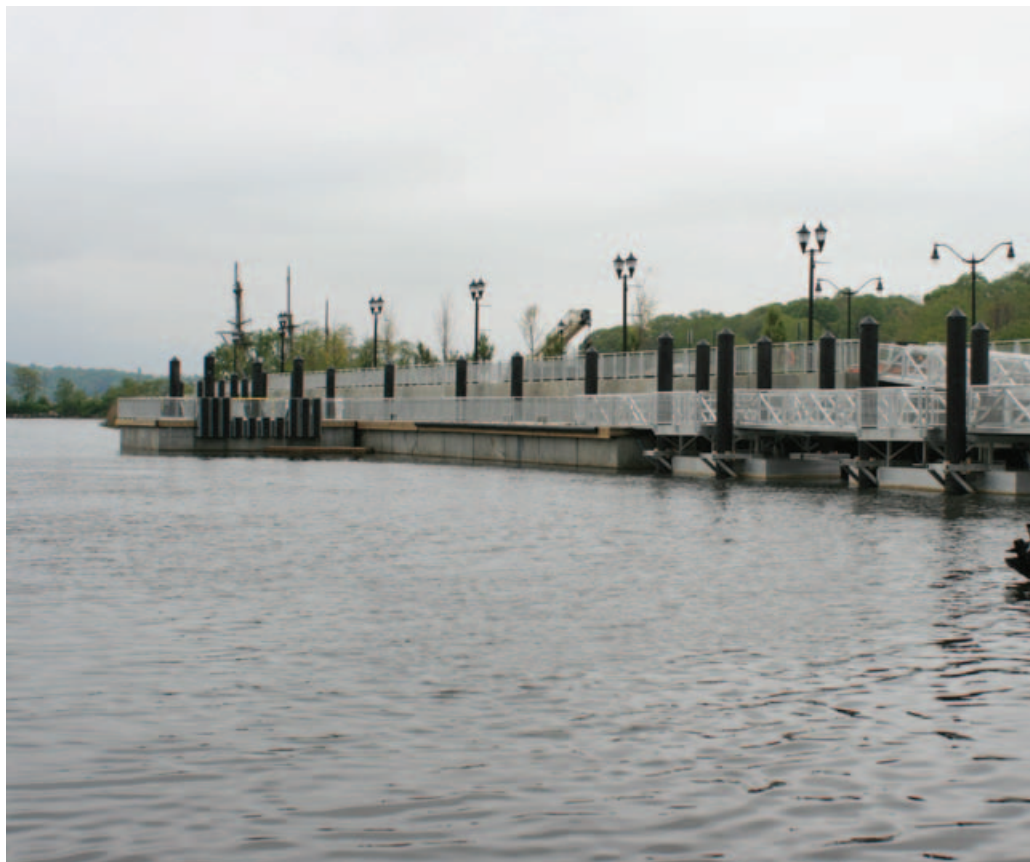
Below: The completed project with gravel parking and lighting beyond the new SSP bulkhead. The new concrete floating dock system by Bellingham Marine Industries is in the foreground along with the aluminum floating landings and gangways by Gator Dock.
