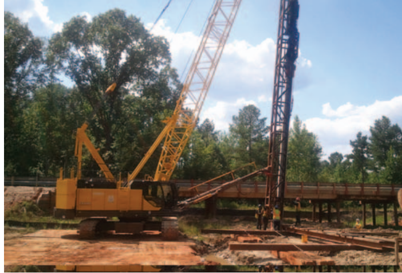
Driving 16-inch test pile in Attala County on Hwy 12. There were 10 different bridge sites on this project
