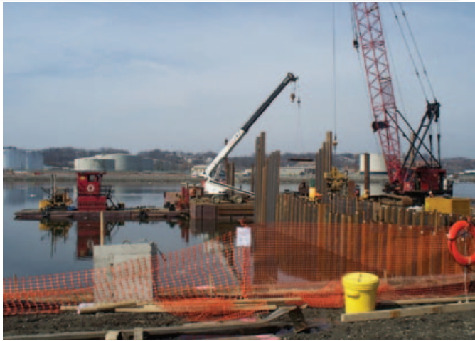
A cofferdam in the Hudson River for the installation of an outfall pipe for the Empire Generating Facility in Rensselaer, N.Y.
