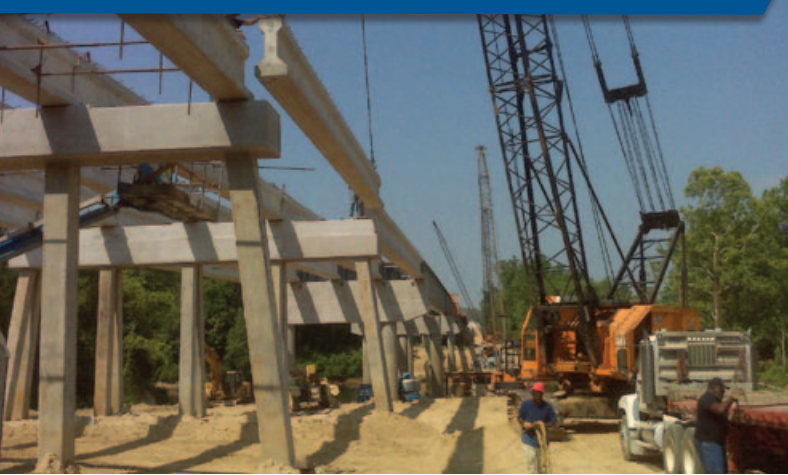
Hanging beams in Marion, Co. for a bridge over the Pearl River on Hwy 43
