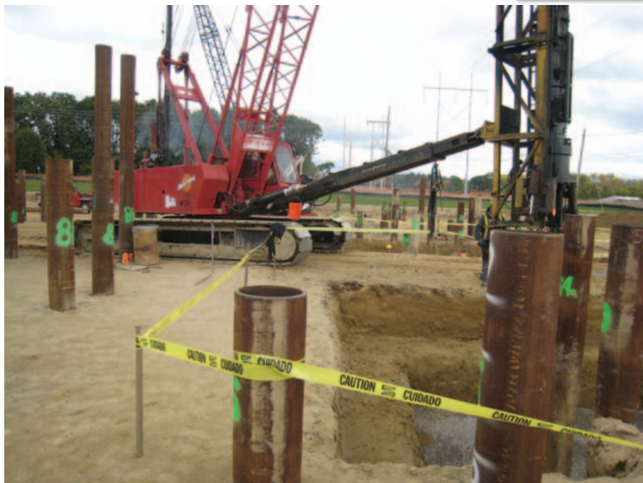
Steel pipe piles used in the redevelopment of an existing commercial lot in Dedham, Mass.
