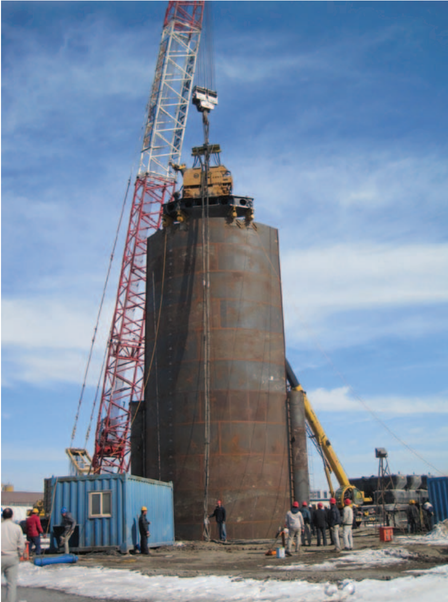
APE China Managing Director, David White, standing next to 37-foot sheet pile prior to test driving
