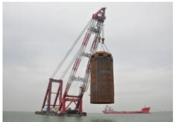
The final pile of the project being transported to the drive location
