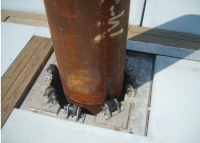
Left: Using a HDPE sleeve protects steel pile driven in salt water Right: The steel pile before the HDPE sleeve is placed over the pile Opposite: HDPE sleeves were used at Yacht Club Costa Smeralda in the British Virgin Islands
