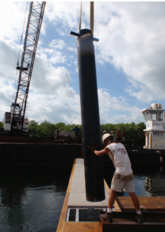
Below: The Ocean Reef Club Marina docks in Key Largo, Fla. feature a telescoping pile system for 80-foot finger piers — a first for marinas in the south east
