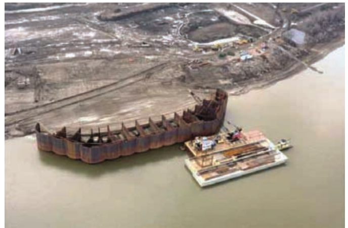
Figure 9. Cates Landing Dock, 2/2012
