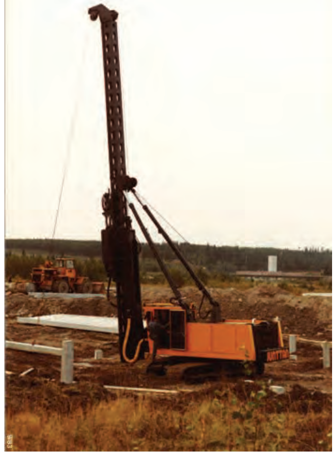
Junttan's fully hydraulic PM20 pile driving rig Photo courtesy of Junttan Oy
