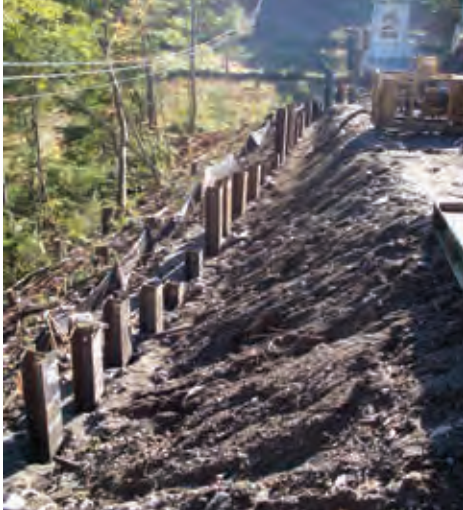
Installed HP12x53 stabilization piles along the north side of the west approach embankment
