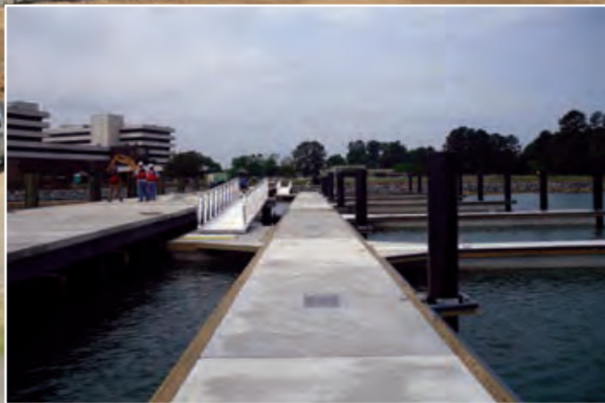
The top of Main Pier 45 was removed, damaged sections were restored, timber pile and caps were replaced, new steel girders were set on top and a pre-cast deck was installed
