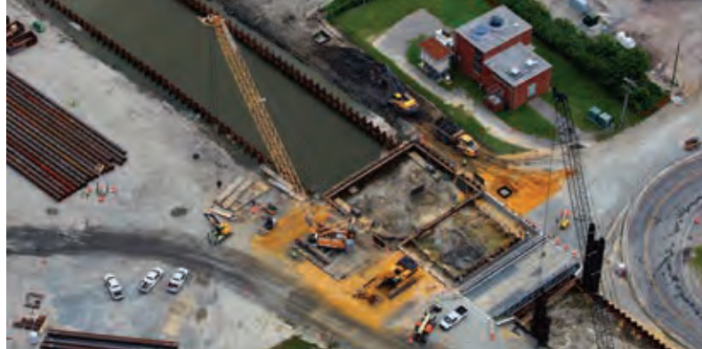
Aerial view of the interface of the Approach SOE (dry) and Dredge SOE (wet). The temporary vehicle bridge is installed in the lower right corner of the picture.
