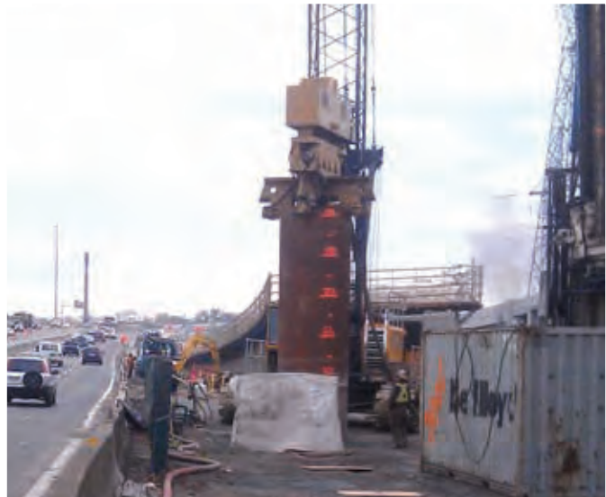
Initial vibratory installation of 1.83-meter diameter open-ended piles, subsequently driven using D-100-42 to design penetration, for flyover foundation on PMH1 Upgrade project
