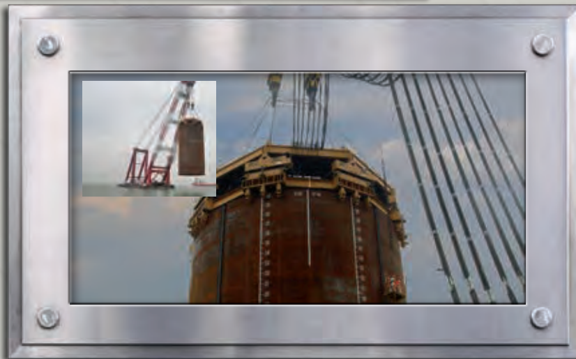
The first pile for the Hong Kong Macau Zhuhai Bridge in China. Inset: The final pile for the Hong Kong Macau Zhuhai Bridge being transported to the drive location. APE won a 2012 PDCA Project of the Year Award for their innovative Octa-Kong system.
