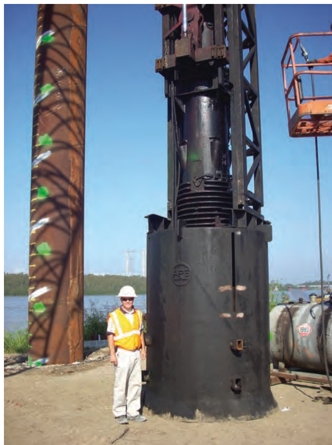
Robert next to APE D80-23 for driving 60-inch pipe piles for Temporary Bent 1E at Audubon Bridge, Louisiana (2008)
