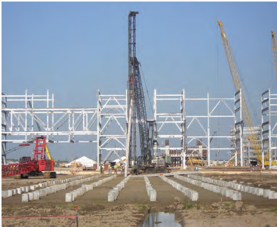
Concrete piles like these, along with timber and pipe piles, made up the 10,204 piles used on site of the Diamond Green Diesel Project
