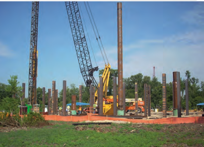
Test pile site (30-inch open-ended pipe piles) at West Closure Complex in New Orleans, La. (2009)
