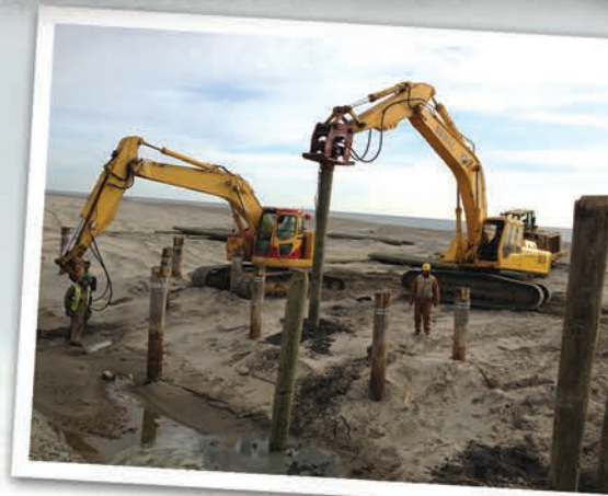
Taken in Avon-By-The-Sea, a municipal boardwalk replacement as a result of Superstorm Sandy
