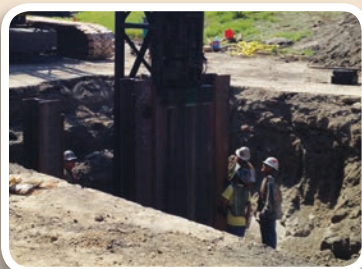
Chris Hill Construction, the foundation contractor, is using a single-acting diesel hammer to install a combi-wall
