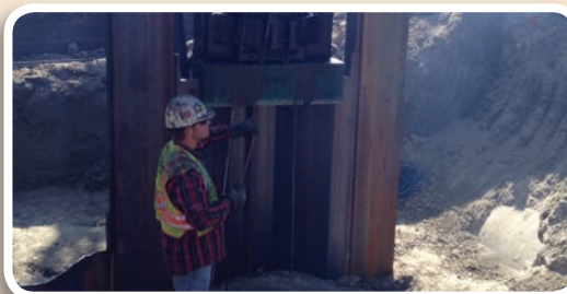
By properly placing and installing the combi-walls, any liquefaction and/or lateral spreading of soil should be minimal
