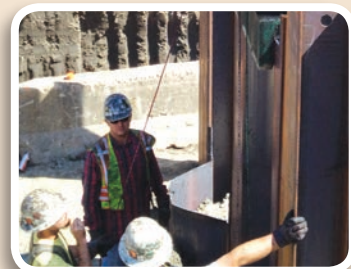
The system consists of three 14-inch by 73-inch H-beams combined with two AZ19-700 double sheet piles between the beams
