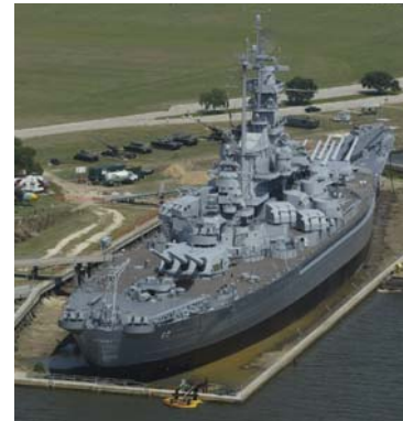
COVER: Restoration of the USS Alabama Battleship, Mobile, AL. Photo: Jordan Pile Driving Inc., Mobile, AL.
